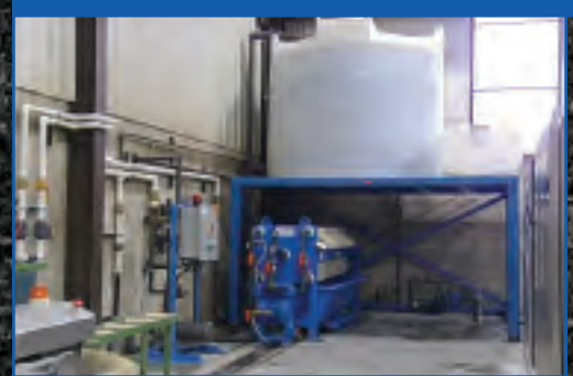
Water treatment system
